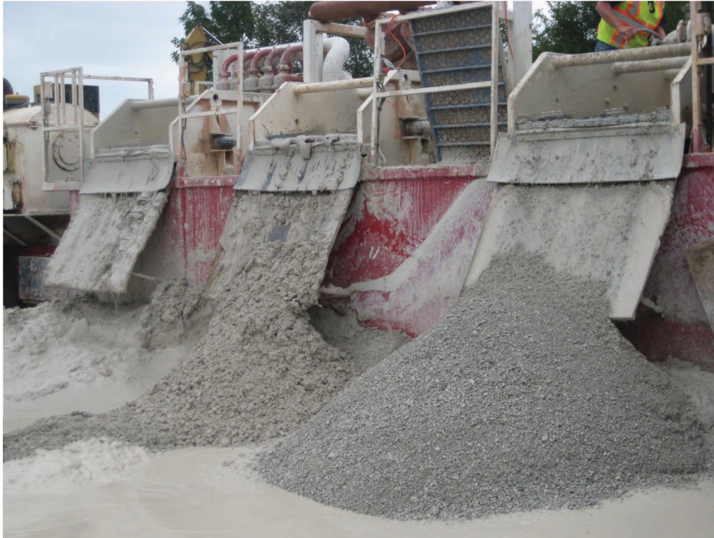
A three-stage drilling fluid recycling system.
