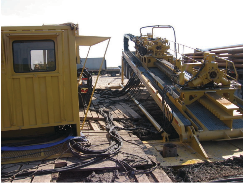
A modern fully hydraulic HDD drill rig with separate drill cab and power unit (hidden behind the drill cab).
